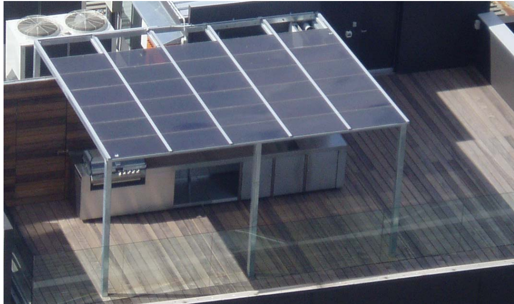
Photo: Some of the Photovoltaics on the Szencorp roof (installed by Going Solar)
