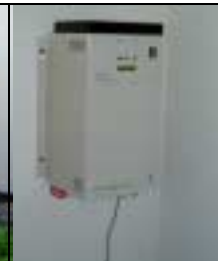
Inverter for connecting the PV panels to the grid power
