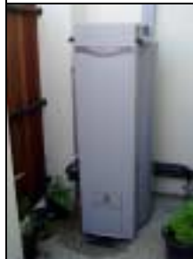
Solar hot water storage tank
