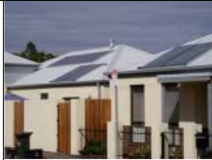
Solar Hot Water and Photovoltaic panels – note the neat appearance and absence of roof tanks
