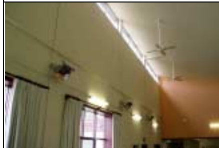
High ceilings and heating problems (Note the lights on in the daytime)
