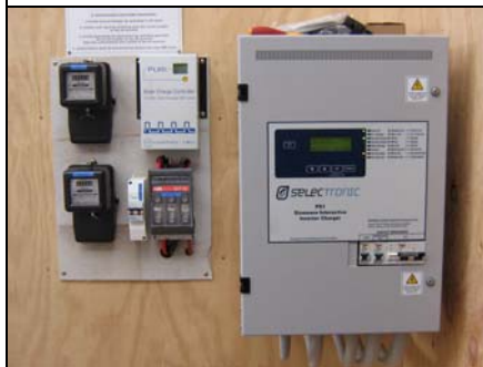
Controls and Inverter/Charger
