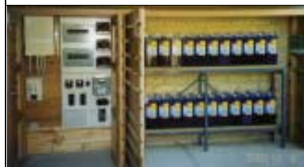
Control system and batteries at the Earth Studies Centre
