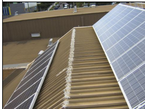
PV Panels on Roof
