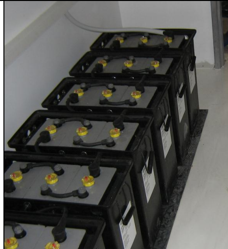
Batteries in leak-proof containers in ventilated room
