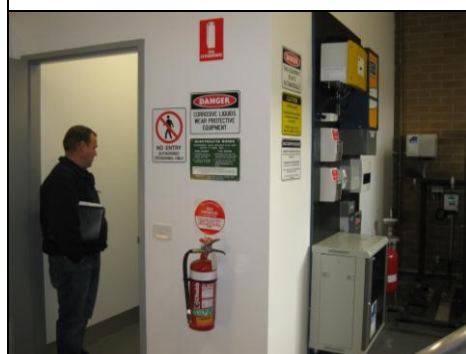
Dedicated Battery Room and Control Equipment
